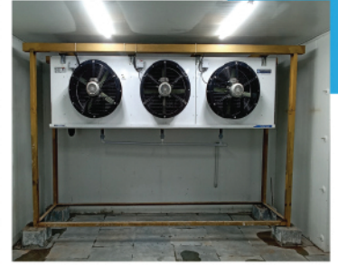
WALL MOUNTED BLAST CHILLER EVAPORATOR
